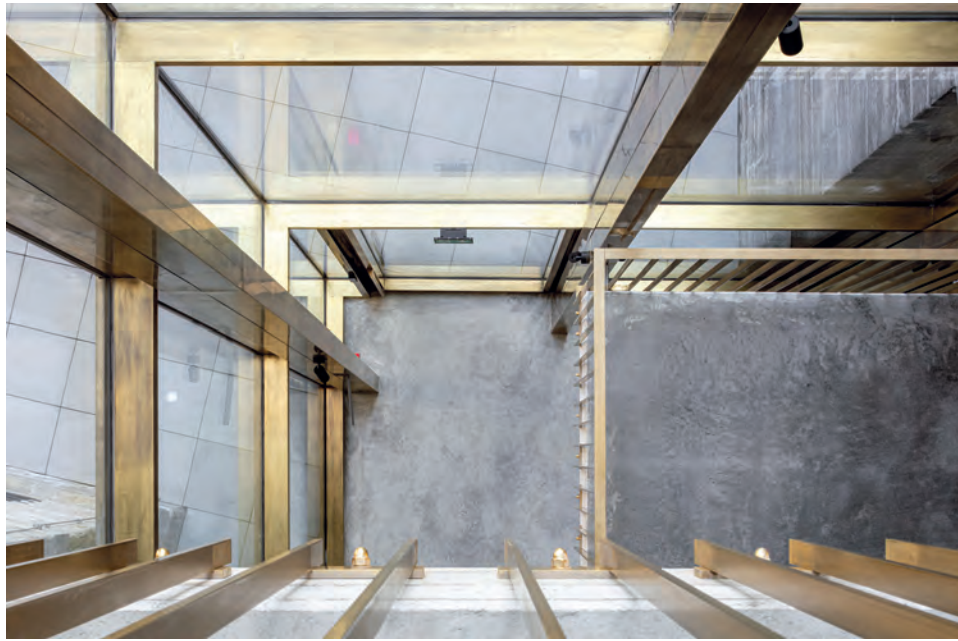
The towering glass front around the new entrance is a mullion-transom construction made using VISS.
