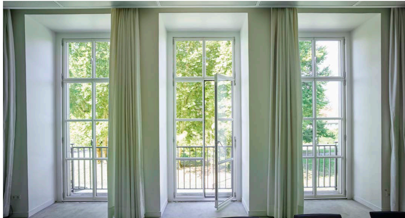
The three window doors in the meeting room of the council groups (Europazimmer) were reconstructed using the Janisol Arte 2.0 steel profile system, following the example of the original fenestration of the 1950s.
